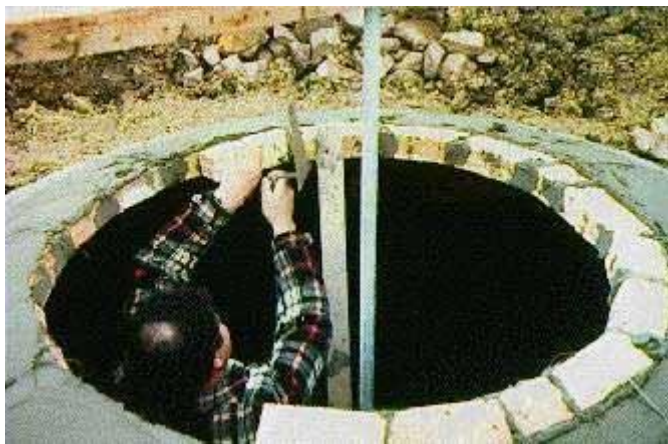
Figure 3: Fixed-dome plant in Tunisia. The final layers of the masonry structure are being fixed.
